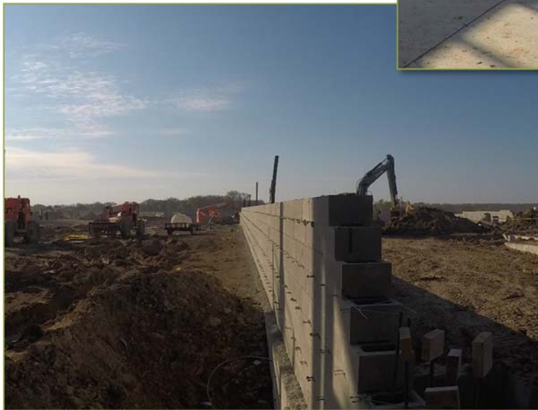
Preparing to pour 2 nd floor at Area B, Inside look at Cafeteria and CMU wall along loading dock area.
