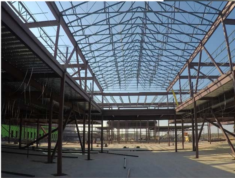
Exterior studs and sheathing being installed, classroom area "D" steel going up, and trusses at Main entry in place
