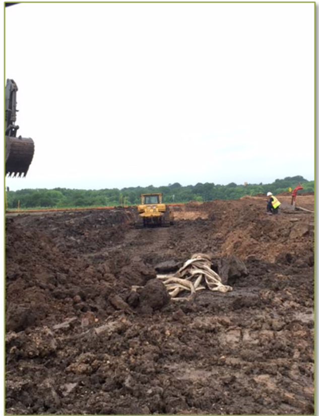
Digging out detention pond on Northwest corner of site. Moisture conditioning the main building pad along the west side of the building.
