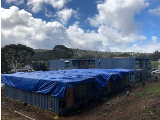
Building B first floor on site, weatherproofed, ready to weld and secure
