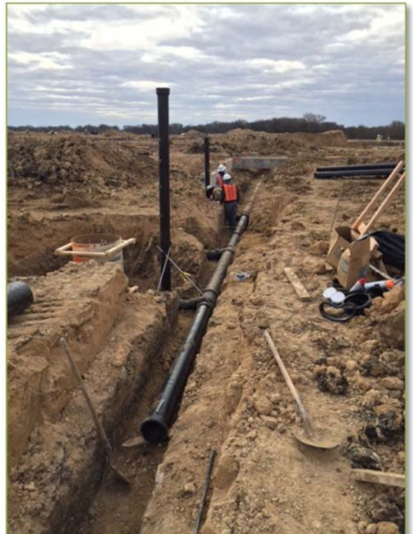
Grade beam form work at Area B underway. Sanitary sewer line at being installed at backfilled in Area K and J.
