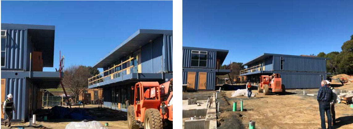
Buildings A and D are set and on site work is underway
