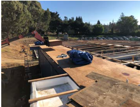
CLC Modulares- Rain protection removed to install electrical connections and above ceiling ductwork
